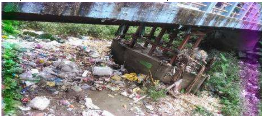
Plate 27: Presence of garbage on river bed. Due to the non-presence of the dumping ground in Falakata, the pollution related to garbage is increasing every day. Along with this, illegal rearing of pigs in the town alongside the river Mujhnai, river Saptana and River Jampui has also led to river pollution. Not only this due to the continuous dumping of waste materials in those rivers, the river base is also raising creating blockage
