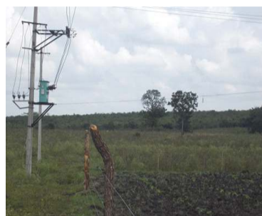
Individual solar fence & lighting at crop land near Metikuppe village. Photo: vishwanatha HR
