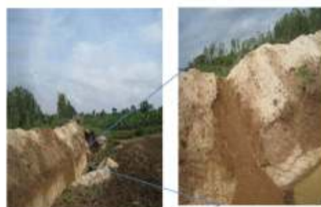
Loose soils sliding into trench at Kademanuganahalli village forest boundary Hunsur Kaluk. Photos:vishwanatha HR
