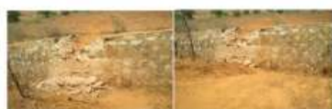
Metal trench damaged by elephants at Tibet camp near Gurupura
